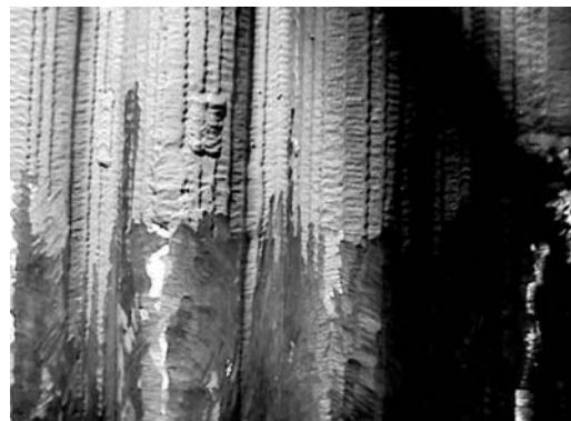
Fig. 12.23 Repair welding can be performed on the corroded waterwall overlay by grinding followed by overlay welding. An alloy 625 weld overlay on the waterwall after 10 years of service in a RDF unit. Shown in the photograph are two tubes and three membranes.
