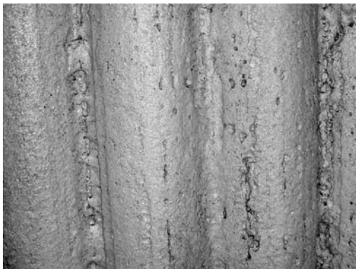
Fig. 12.22 Pitting attack is the common mode of corrosion of alloy 625 weld overlay on the waterwall. Shown in the photograph are three tubes and three membranes.
