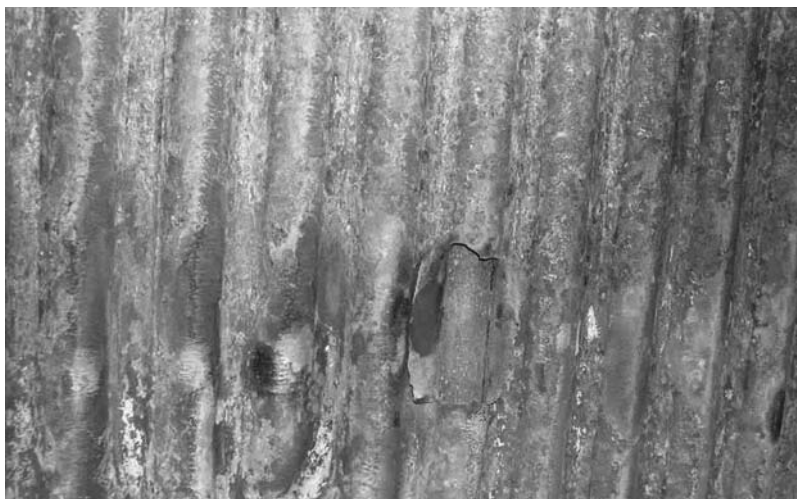
Fig. 12.4 Carbon steel waterwall suffering blown tubes due to high wastage rates resulting in significant tube-wall thinning after 8 months of service in a WTE boiler. Courtesy of Welding Services Inc.
