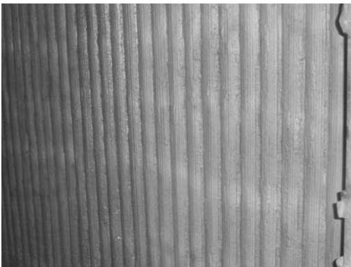
Fig. 12.18 General view of an overlaid waterwall with alloy 625 overlay in a WTE boiler. Courtesy of Welding Services Inc.
