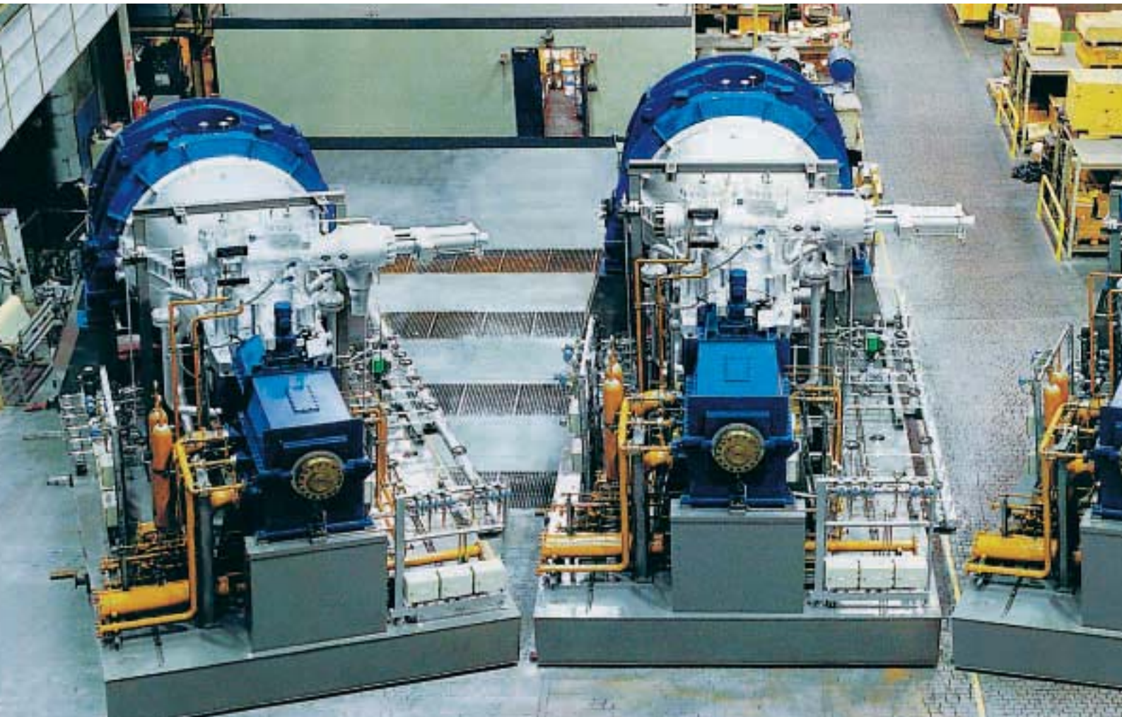
2 Three 38 MW condensing steam turbines for a 300 MW e combined-cycle power plant
